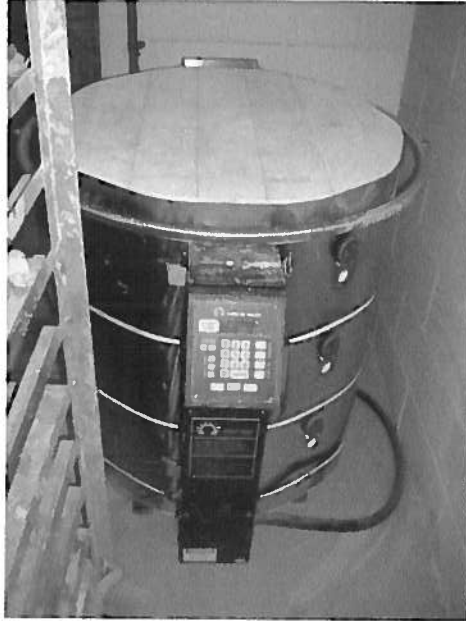
Photo 2: Suspected ACMs in the refractory linings of the two (2) kilns located in the kiln room (Room 18) at the Dovercourt Recreation Complex. (August 21, 2009).
