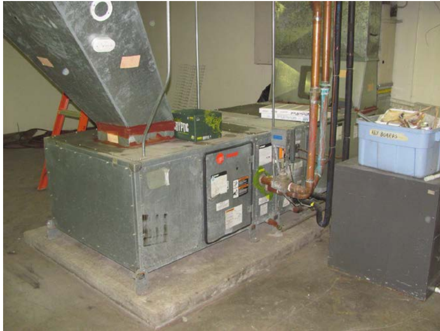
Photo 16: Air handling unit (AHU)
