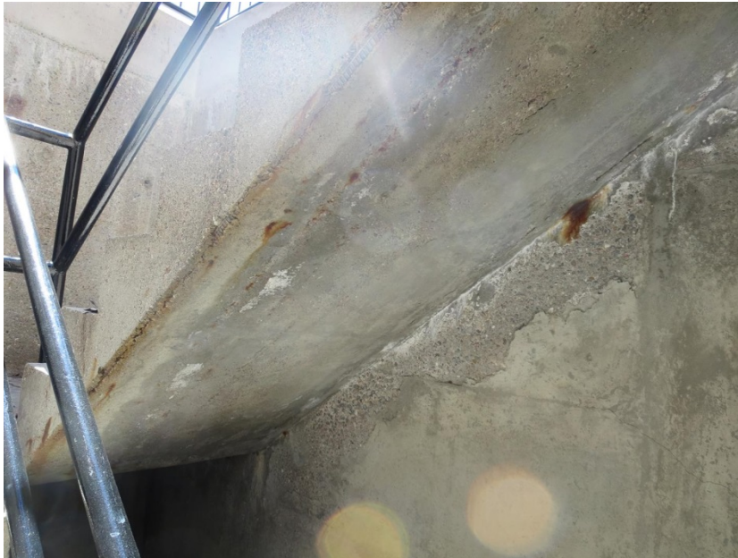
Photo 25: Deterioration at stairs
