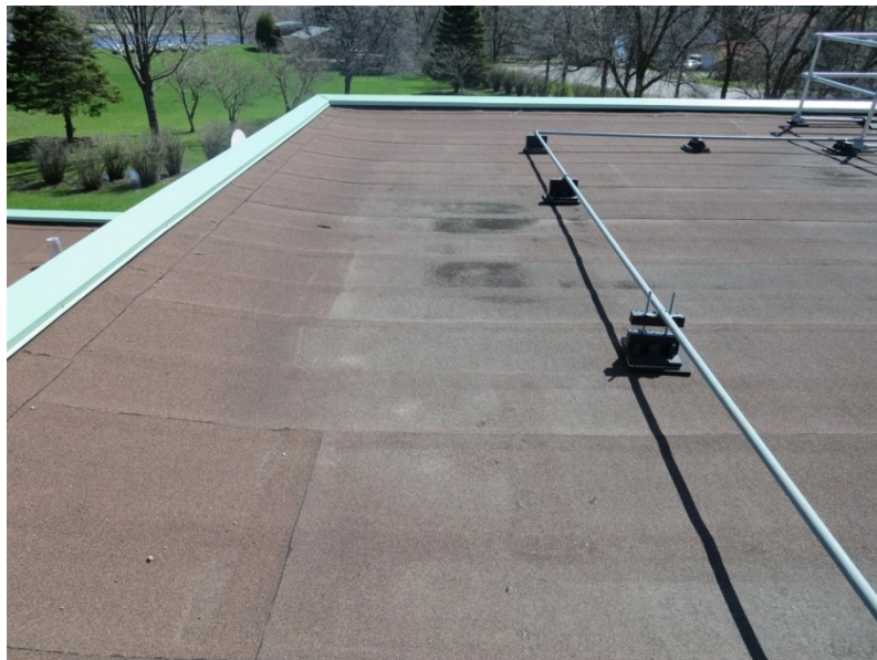
Photo 7: Gymnasium roof – low spot
