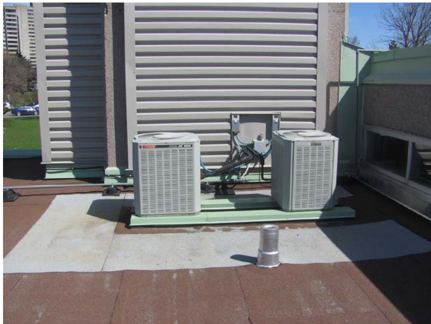
Photo 17: Condenser units for AHU
