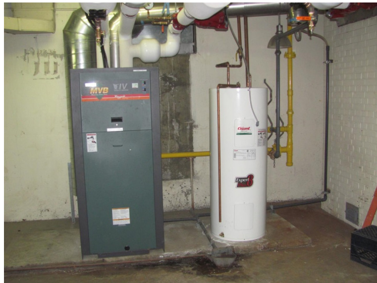
Photo 18: Boiler and water heater
