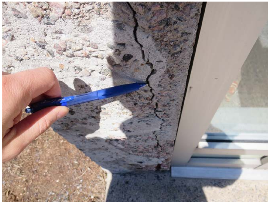
Photo 4: Crack at 50s Club door
