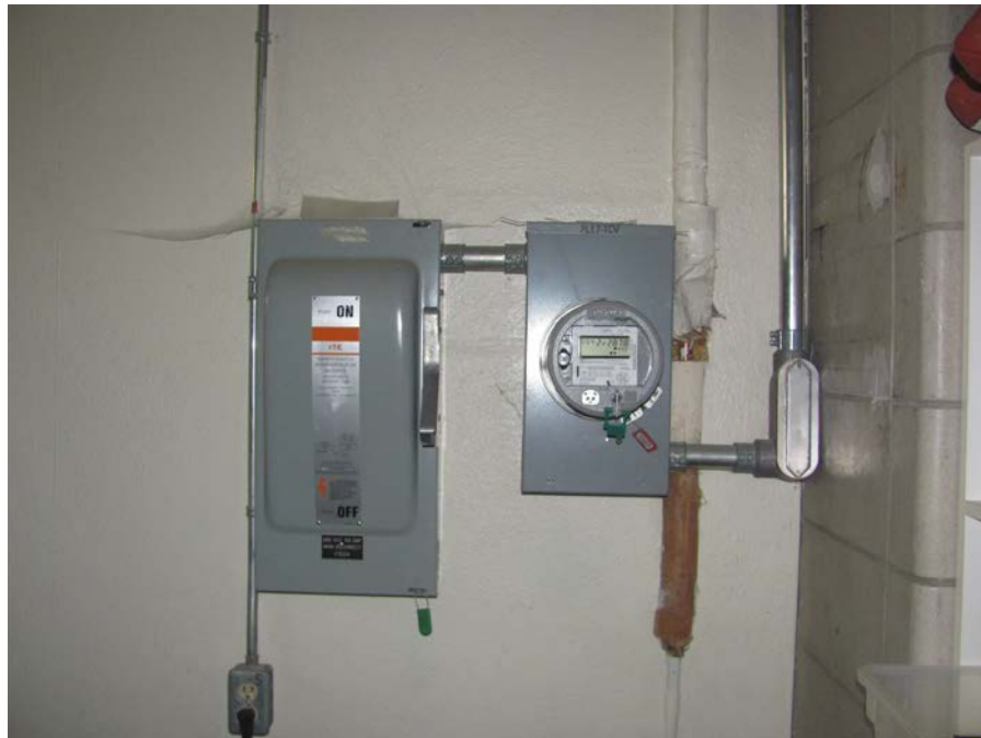
Photo 15: Main electrical switch
