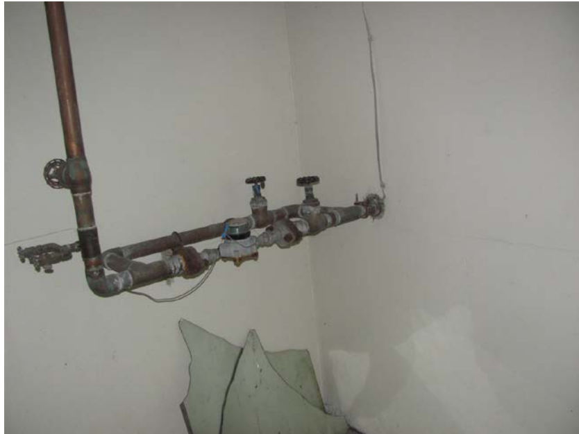
Photo 20: Main incoming water line
