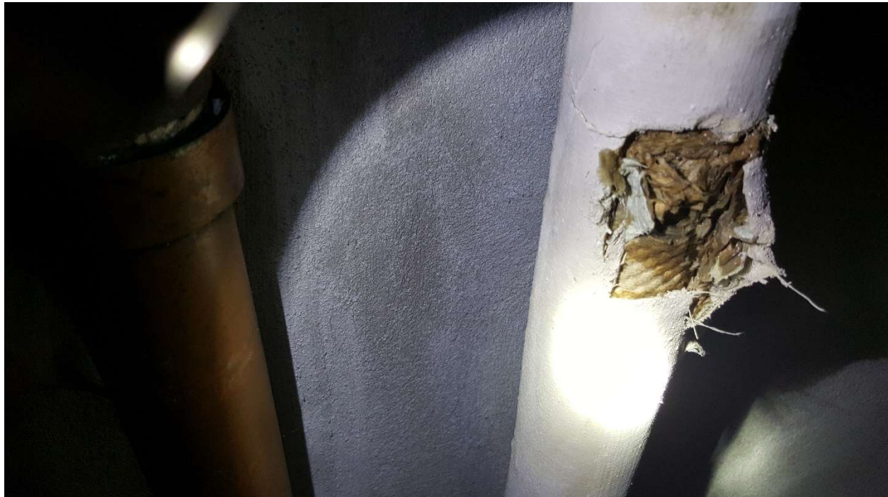
Photograph 9: Friable cardboard wrap pipe straight run insulation which contains 5% Chrysotile asbestos (DST Sample 12A-C) were observed in the basement south-east and south/middle storage rooms.
