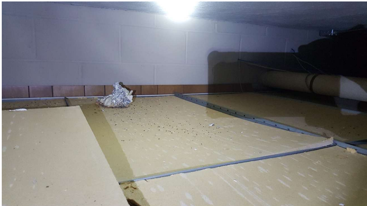
Photograph 10: Rodent feces and signs of rodents feeding were observed in the basement south-east storage room above the ceiling tiles.
