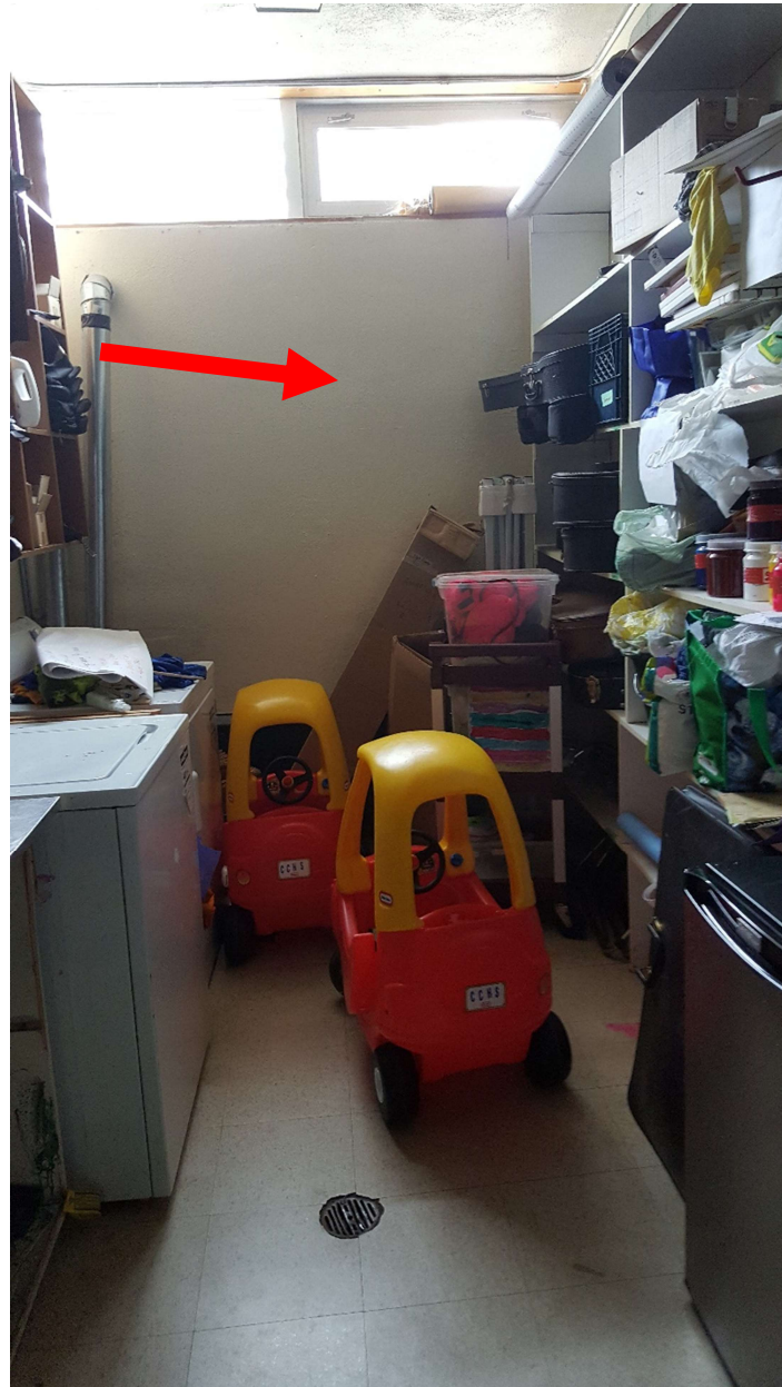
Photograph 6: Non-friable rough textured plaster, which contains 0.5% Chrysotile asbestos, observed on the walls of the rooms north of the gymnasium.
