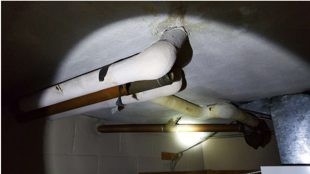
Photograph 7: Non-friable rough textured plaster, which contains 1% Chrysotile asbestos, observed on the ceilings of all basement storage rooms.
