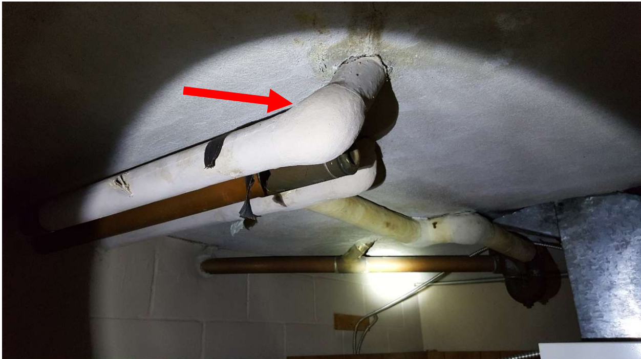
Photograph 4: Friable mechanical pipe insulation fittings which contain 90% Chrysotile asbestos (Seacor Sample SA-9) were observed in the basement south-east storage room above the ceiling tiles.
