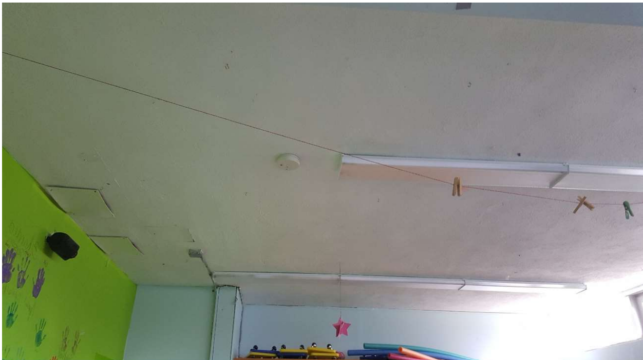
Photograph 8: Non-friable rough textured plaster, which contains 1% Chrysotile asbestos, observed on the ceilings on the main level in the two rooms north of the gymnasium.
