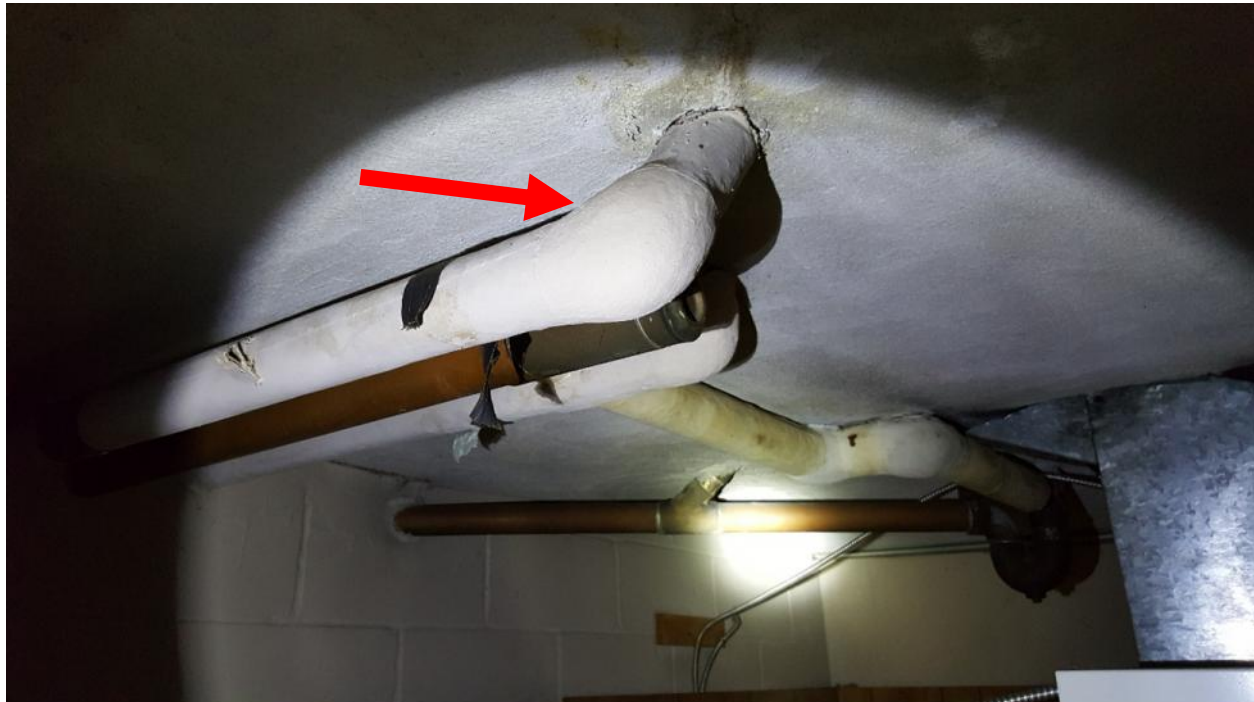
Photograph 4: Friable mechanical pipe insulation fittings which contain 90% Chrysotile asbestos (Seacor Sample SA-9) were observed in the basement south-east storage room above the ceiling tiles.
