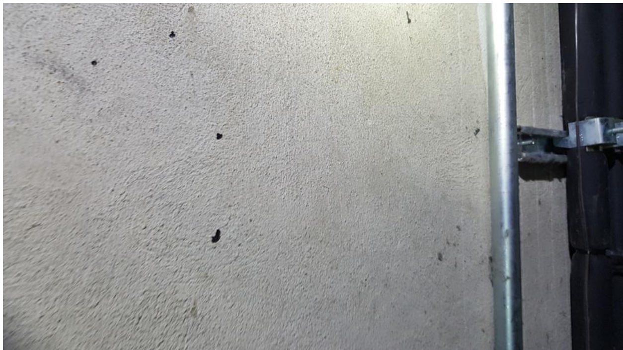
Photograph 5: Non-friable rough textured plaster, which contains 0.5% Chrysotile asbestos, observed on the walls of the former bell tower.
