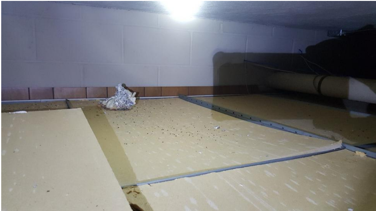
Photograph 10: Rodent feces and signs of rodents feeding were observed in the basement south-east storage room above the ceiling tiles.
