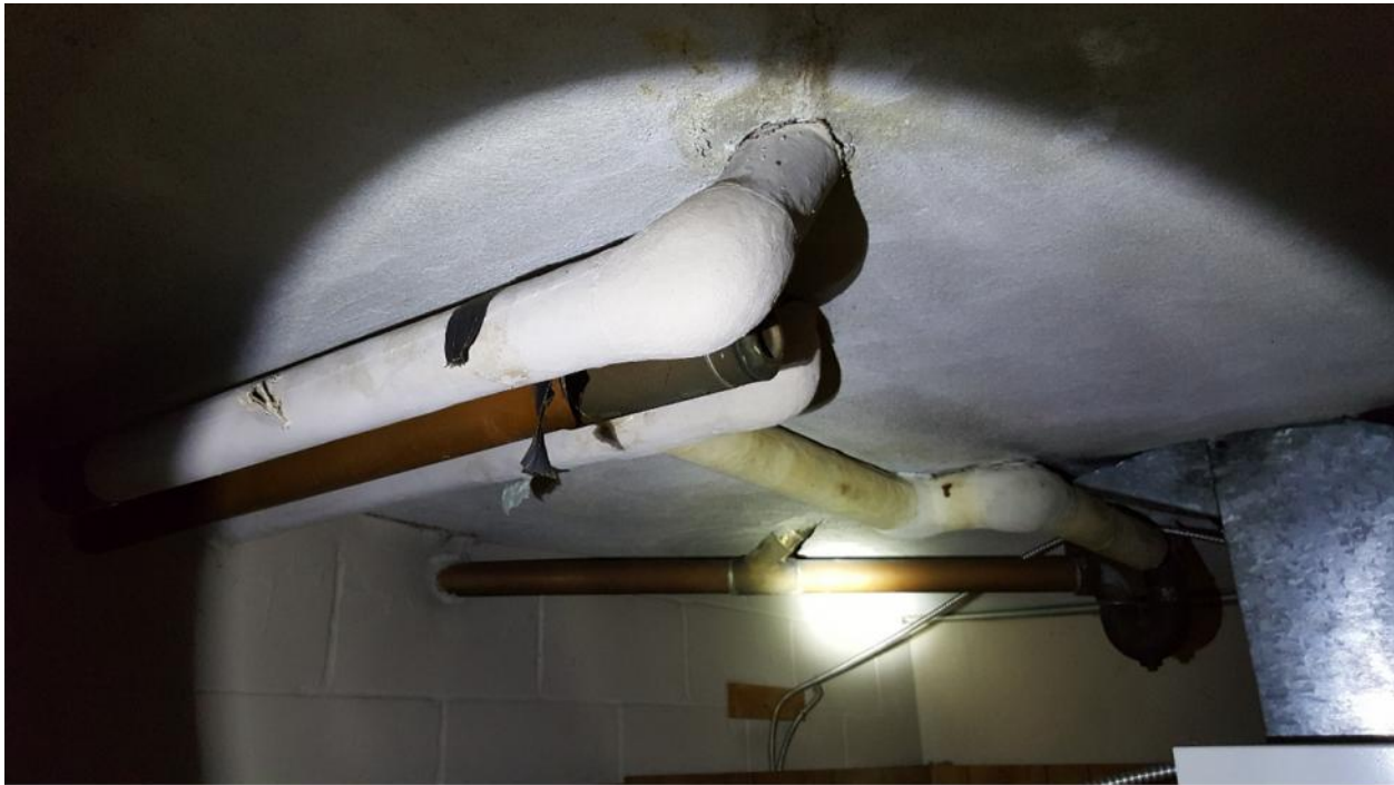
Photograph 7: Non-friable rough textured plaster, which contains 1% Chrysotile asbestos, observed on the ceilings of all basement storage rooms and the basement corridor.
