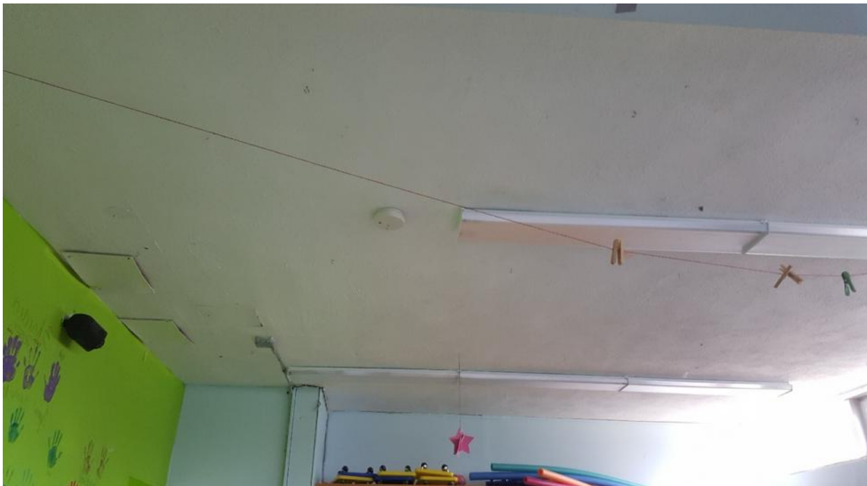
Photograph 8: Non-friable rough textured plaster, which contains 1% Chrysotile asbestos, observed on the ceilings on the main level in the two rooms north of the gymnasium.
