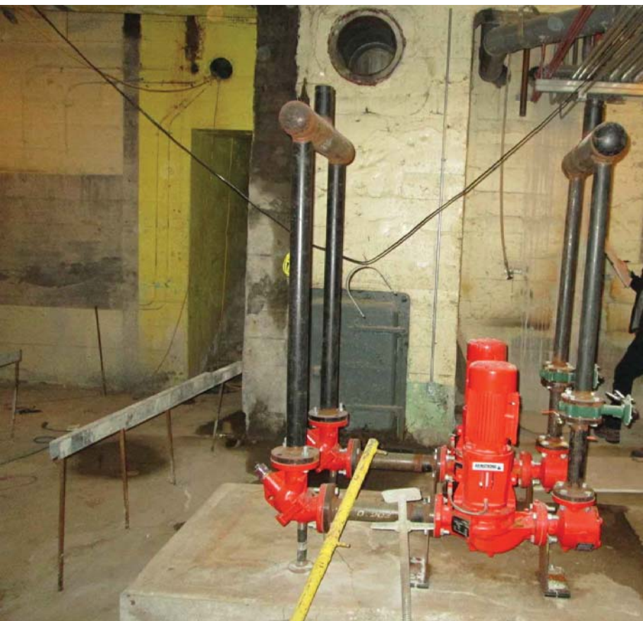
EXISTING HEATING PUMPS
