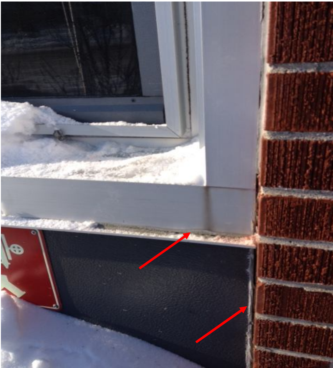
Photo 5 – View of asbestos grey exterior caulking on windows and flashing.
