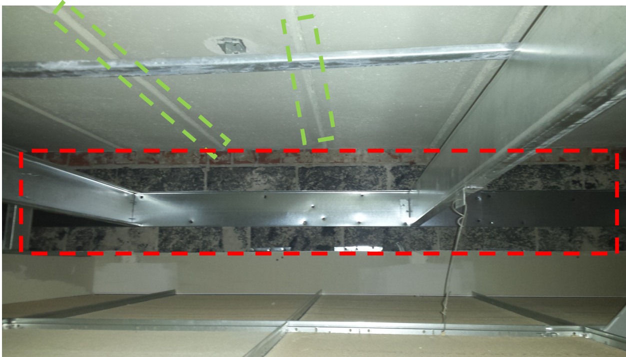
Photo 1 – View of remnant plaster on brick above ceiling grid (Red), and Siporex mortar (Green).
