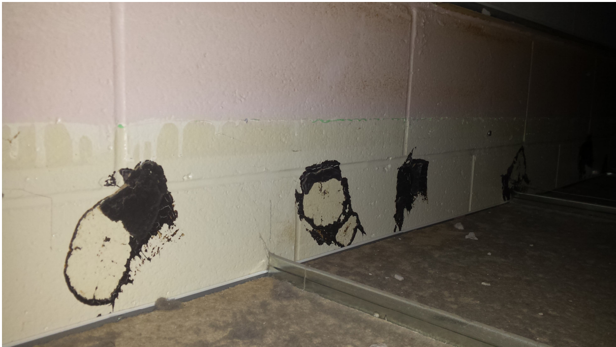
Photo 2 – View of Black Adhesive Pucks on Concrete Block above ceiling grid..
