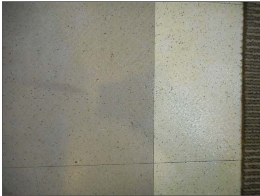
Non-asbestos 12" white and grey vinyl floor tiles with black dots.
