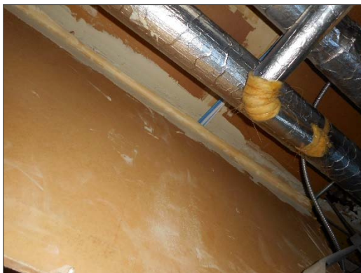
Asbestos-containing drywall joint compound present on drywall wall and ceiling finishes throughout the assessed area (Photo taken above suspended ceiling).
