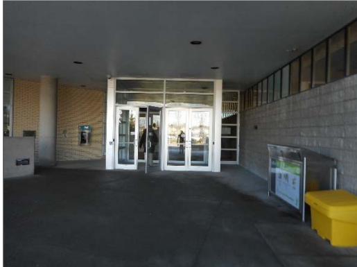
Non-asbestos drywall joint compound present on the underside of the exterior canopy at the main entrance.
