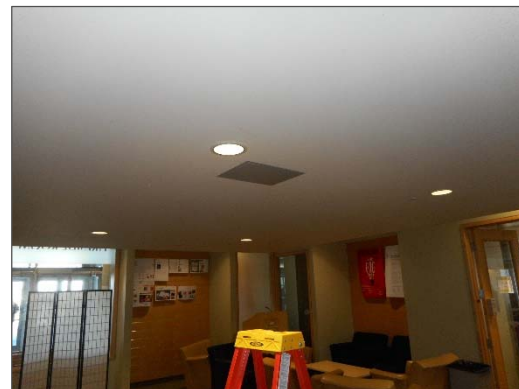
Asbestos-containing drywall joint compound present on drywall wall and ceiling finishes throughout the assessed area.
