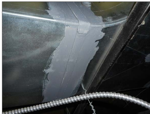
Non-asbestos grey duct mastic.
