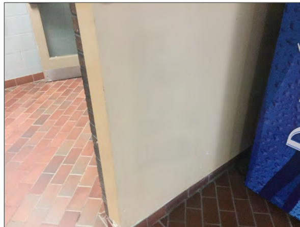
Non-asbestos drywall joint compound on wall.
