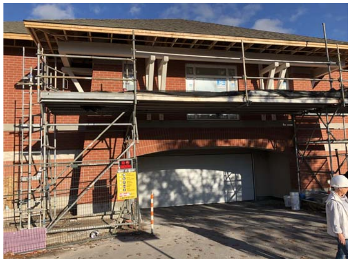
12 Wood Beam & Brackets
