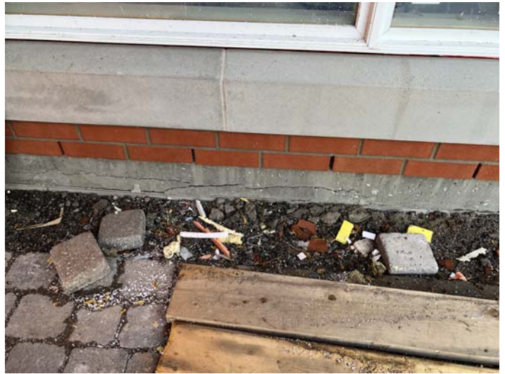
08 Cracks in Concrete Curb
