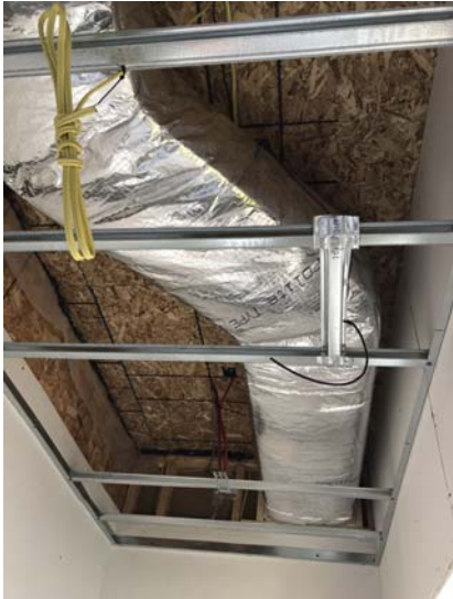
01 Duct in Stor-3
