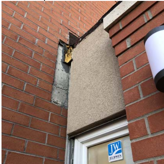
03 Exposed Concrete at Links
