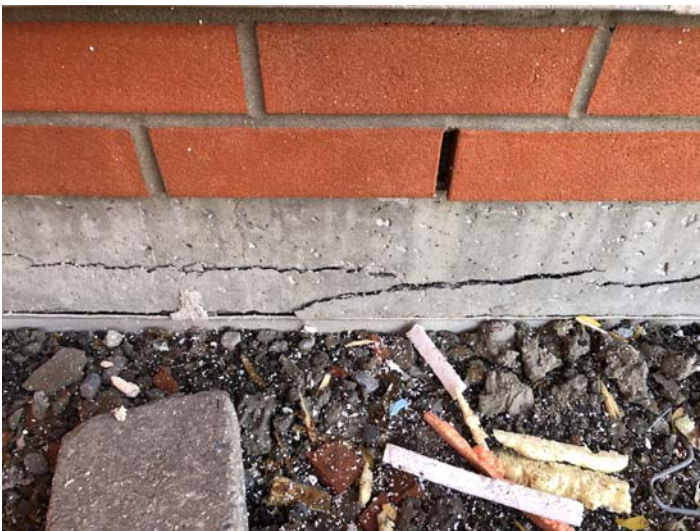
09 Cracks in Concrete Curb
