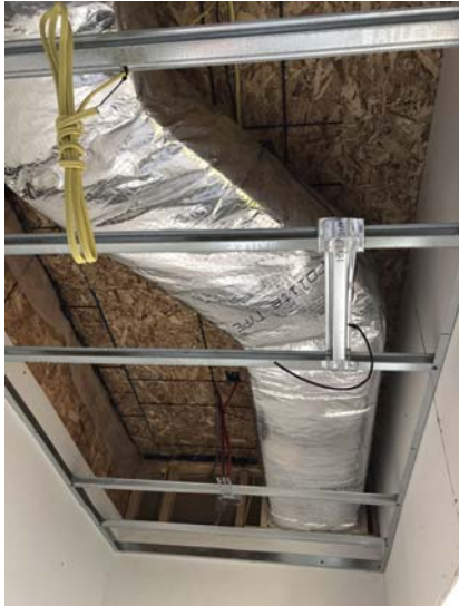
01 Duct in Stor-3
