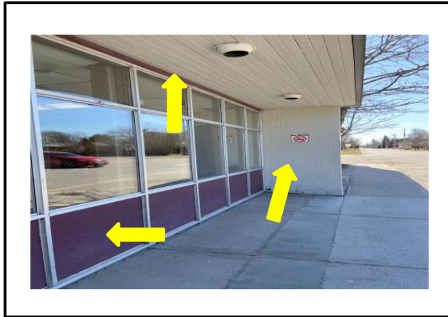
Photograph 5: Exterior Lead-Containing Red and White Paint.
