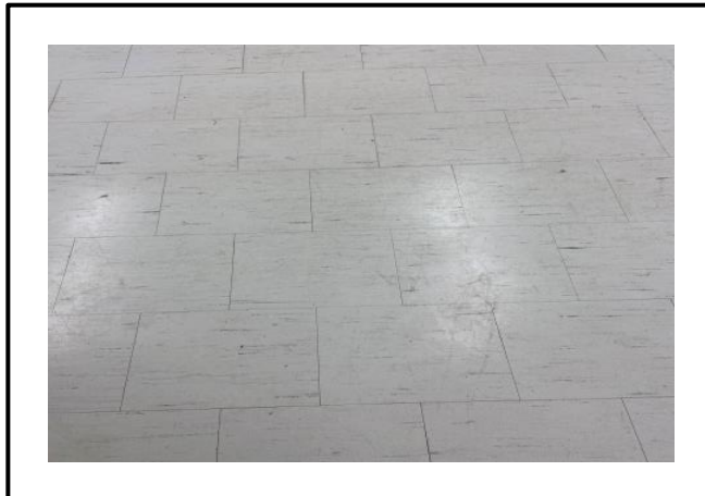
Photograph 3: 12" x 12" White w/Black Streaks Vinyl Floor Ties – Room Next to Main Entrance.
