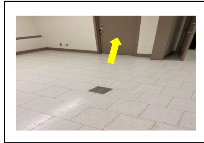
Photograph 6: Lead-Containing Doors and Frames
