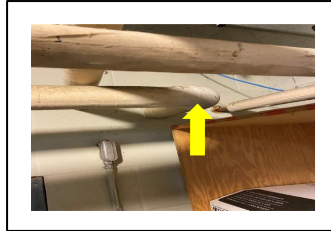
Photograph 2: Parging Cement Elbow – Mechanical Room
